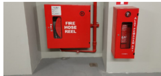
Hose Reel and Fire Extinguisher
