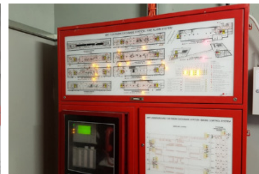
Fire Alarm Panel
